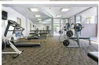
The dehumidifiers of the DS series are also ideally suited for use in fitness areas.
