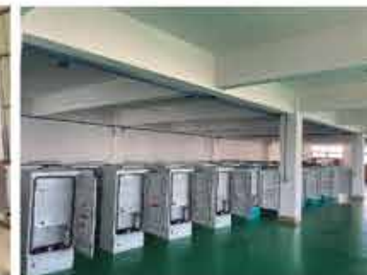
Road Traffic light controller
